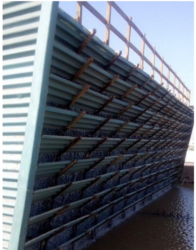
Wooden crossflow tower with corrugated FRP casing.
