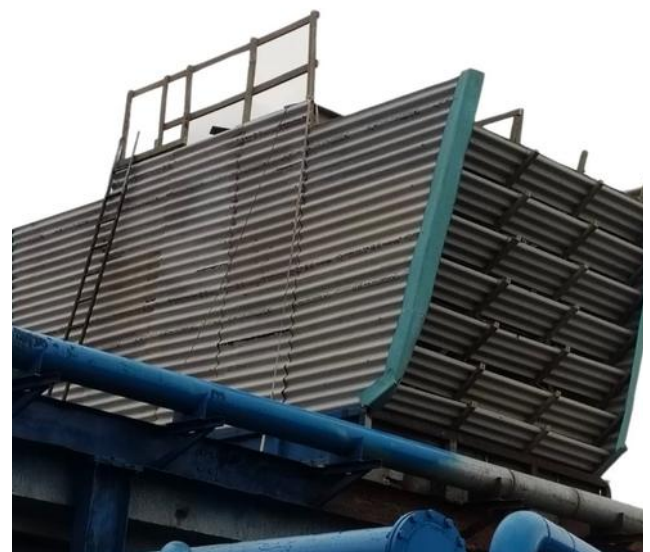
Wooden crossflow towers in service at Indian process plants.
