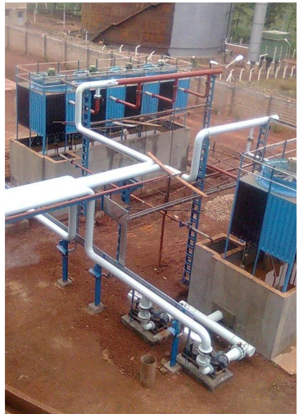
Twin pultruded FRP counterflow towers.
